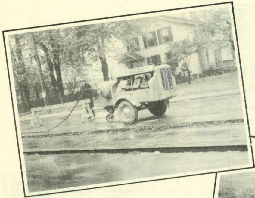
Fig. 6 → Paving crew preparing road bed for binder course to be laid immediately after removal of rail.
