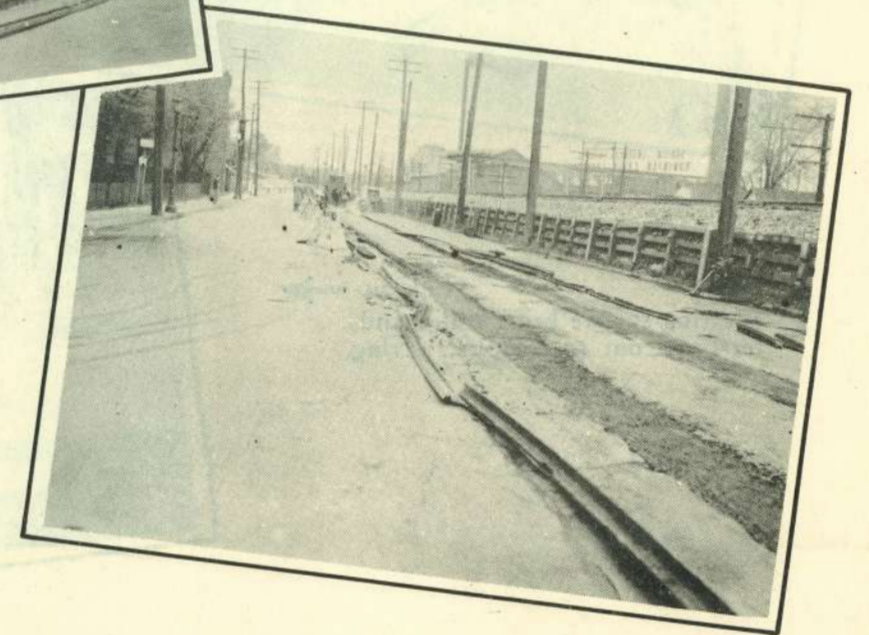
Fig. 20. → Binder course in place and rolled. In congested areas traffic was routed over same before wearing surface was put down.
